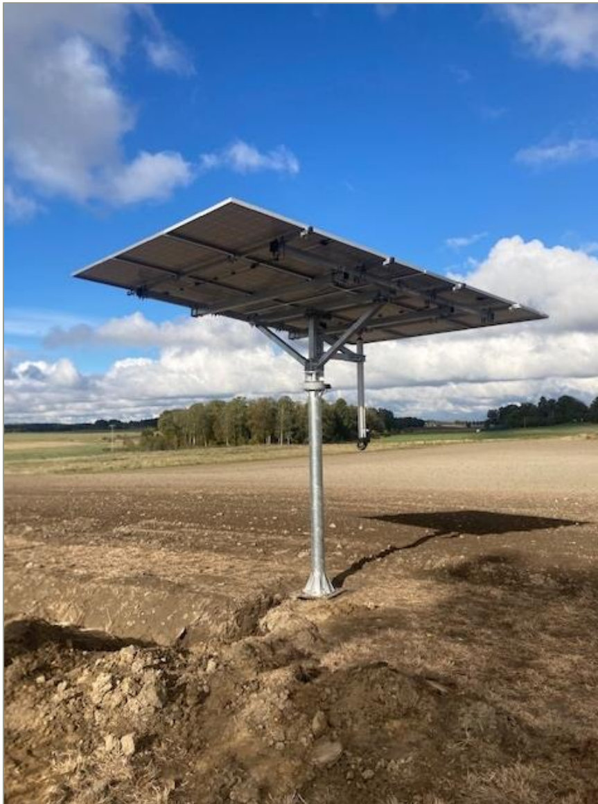
Superstate Solar Tracker installed at Eneby Farm in Stallarholmen, Sweden
